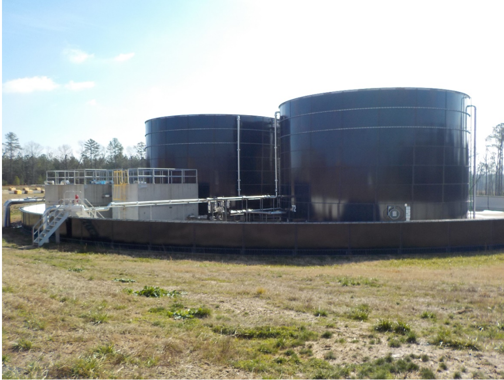
Photo 19 - Leachate tanks looking south
