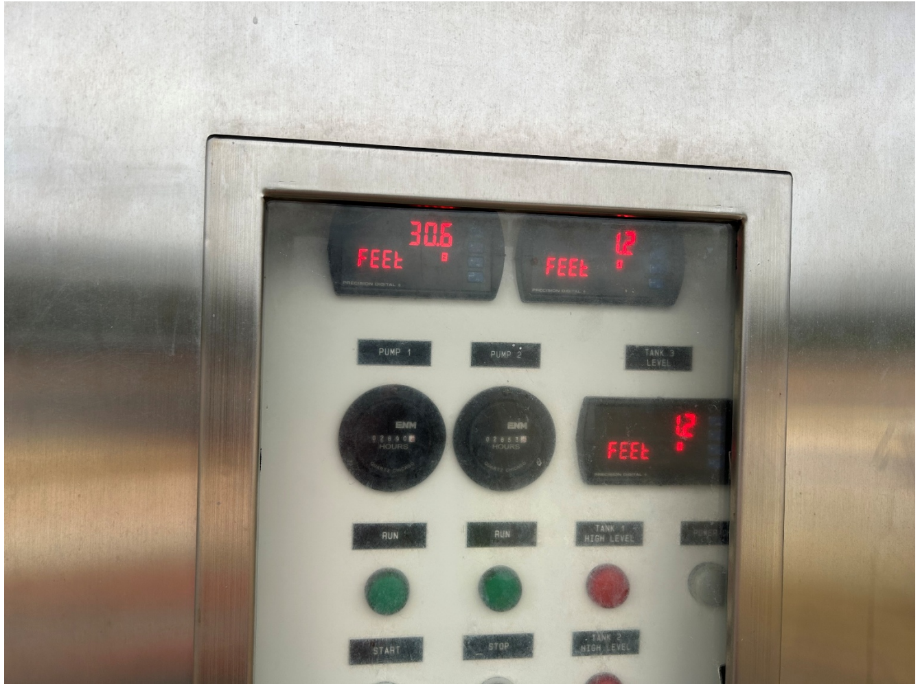
Photo 20 Leachate Tank Levels
