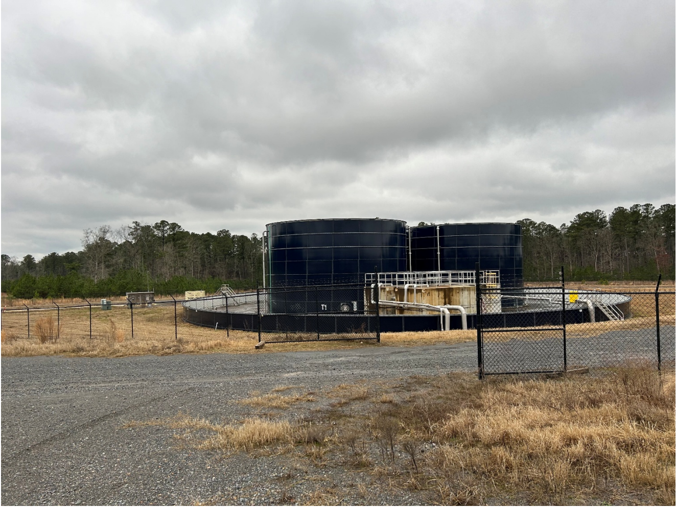
Photo 8 Leachate Tank farm looking south
