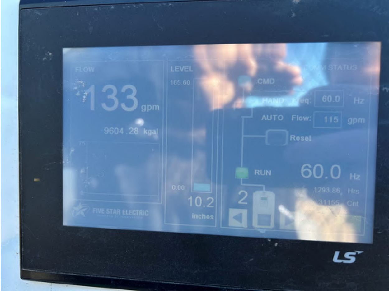
Photo 12 – Sump 6 Read Out
