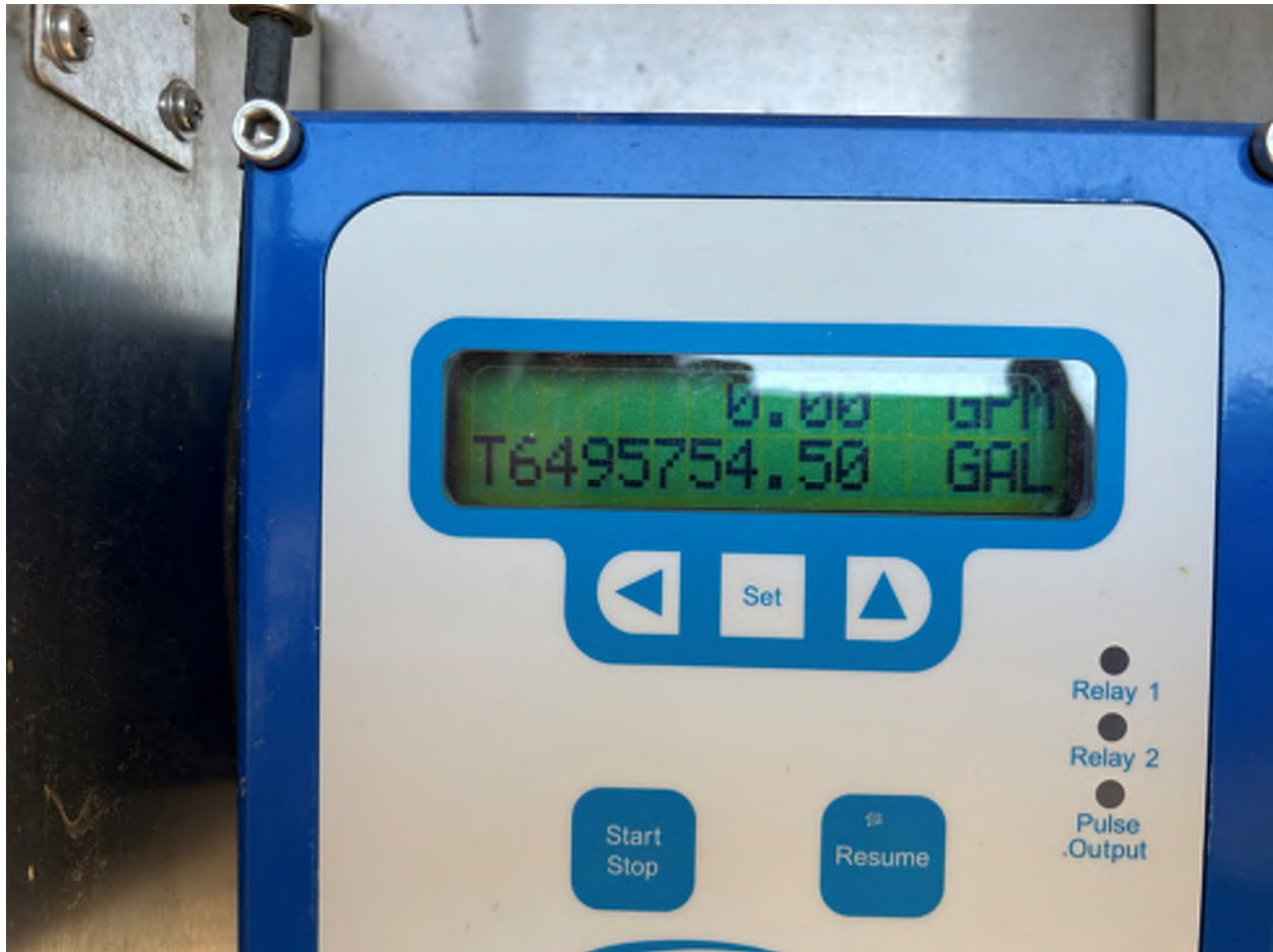
Photo 16 – Leachate Tank Totalizer Read Out
