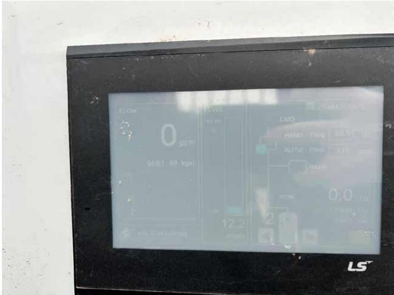
Photo 9 – Cell 6 Sump leachate level readout
