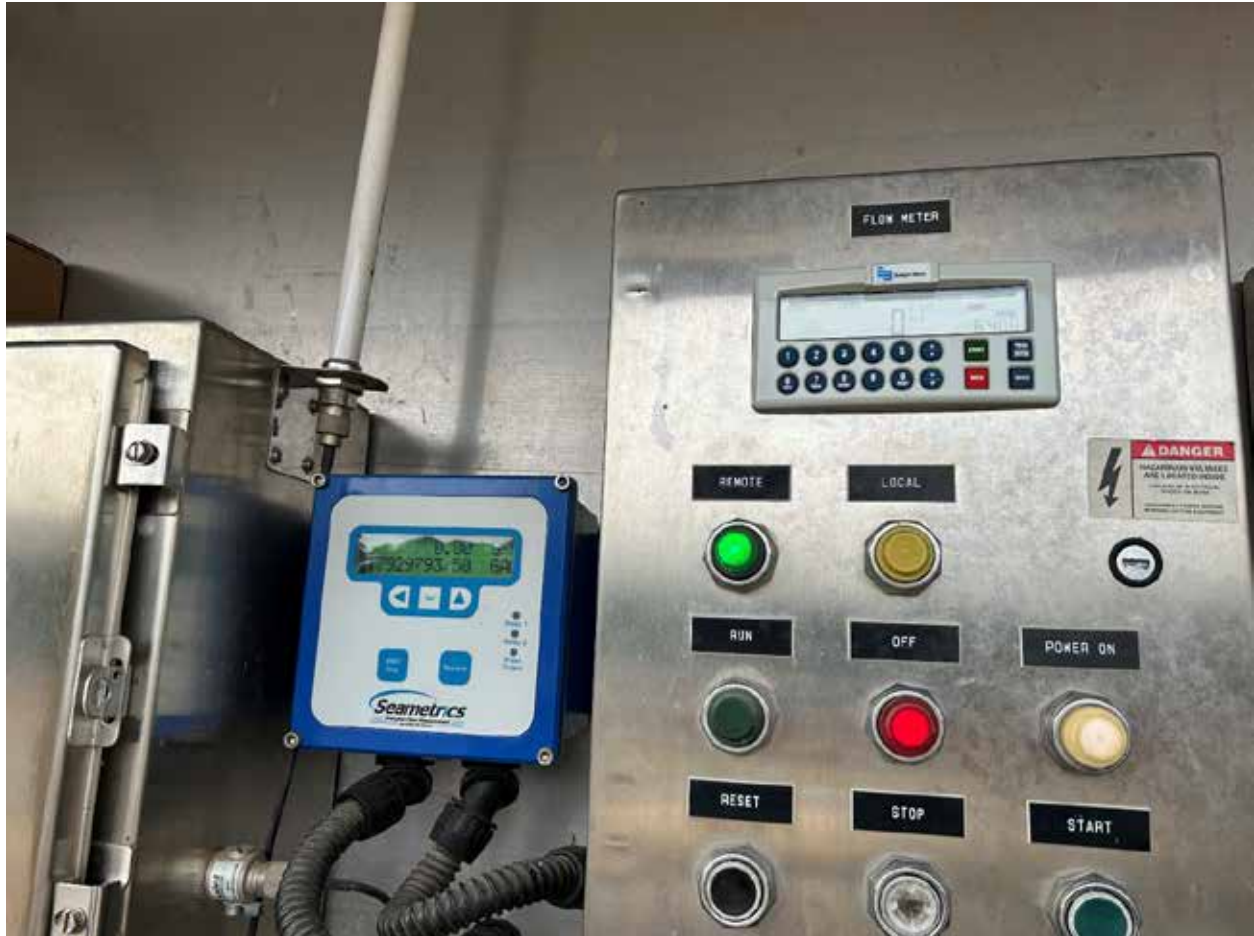
Photo 14 – Leachate tank pump station readout
